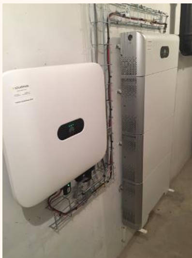
Figure13. 15 kWh battery unit and battery inverter for 1 of the 19 housing blocks
