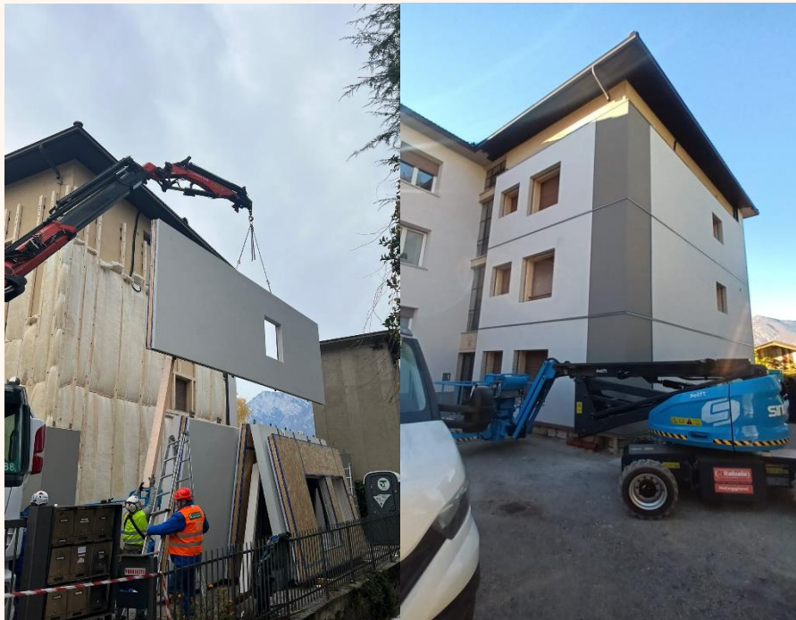
Figure 24. Before and after the installation of the “Renew Wall” retrofit kit in Povo.
