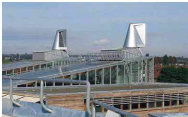
Figure 19: Wind cowls enhancing NV in Nottingham Jubilee Campus (England) [25]
