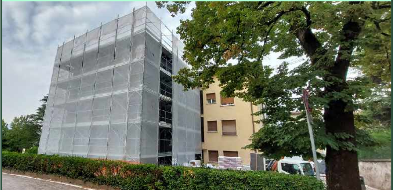
Construction site before the installation of the EPS insulation (ETICS) and RW panels
