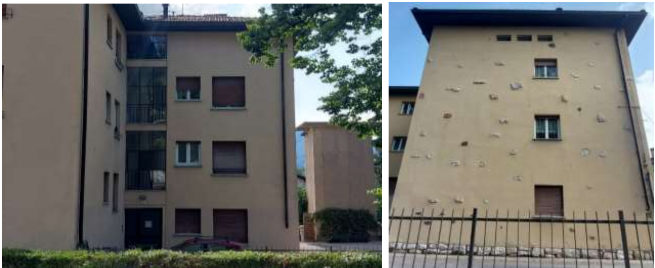
Figure 46. North and East façades before the application of the Renew Wall panels. Source: UNITN.
