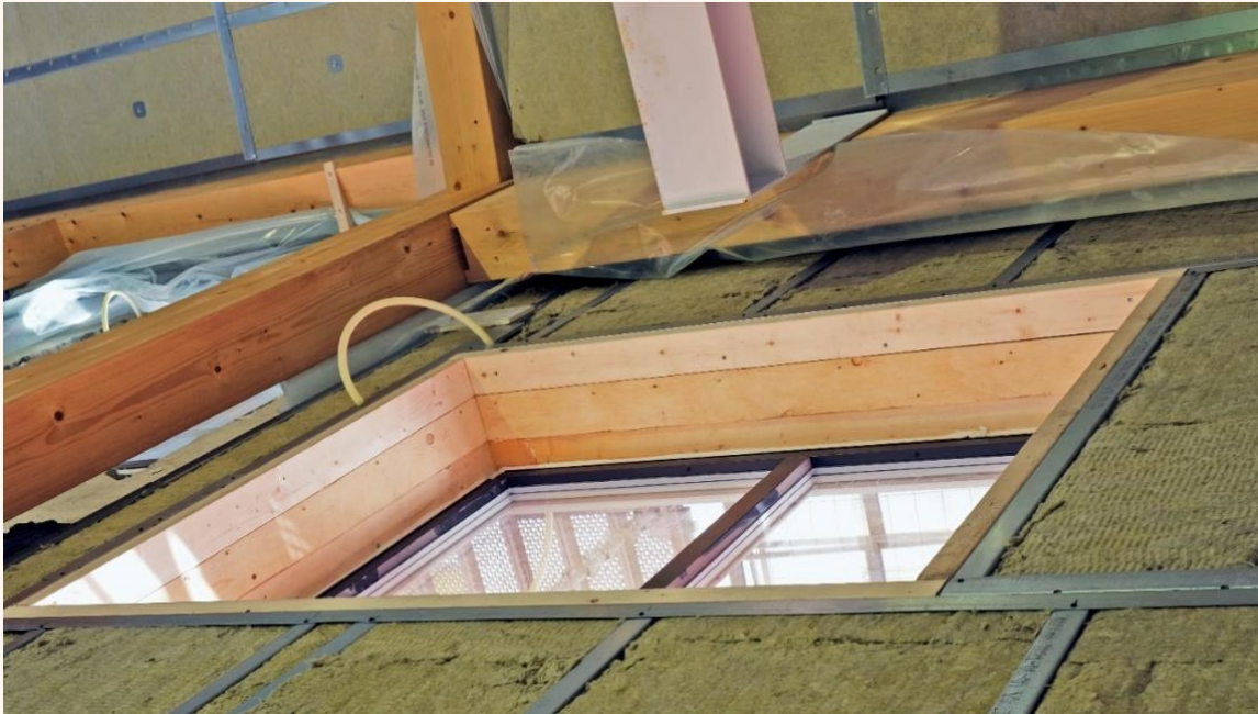
Figure 37. Image of the internal insulation layer in the H-building. The new wood structural system is shown. The gypsum boards, not installed yet, are to be placed between the vertical and the horizontal wood frame. Photo by Nicola Lolli (SINTEF).
