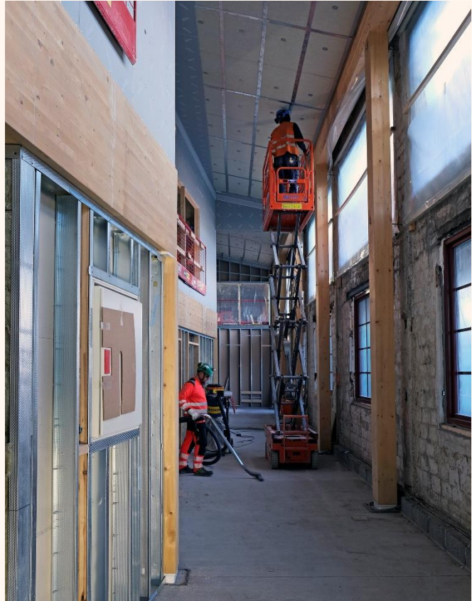
Figure 62. Photo of the exposed façade (right in the picture) and cultural spaces (left in the picture) in the north side of the H-building. Photo by Nicola Lolli (SINTEF).
