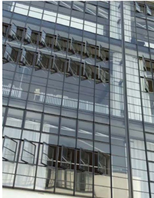
Figure 11: Bauhaus (Dessau-Roßlau) – lined up windows operated by one unique joint actuator [25]
