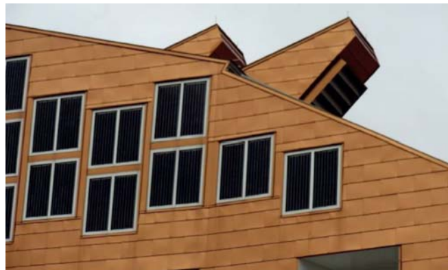
Figure 22: Harm A. Weber Academic Center at Judson University in Elgin (Illinois, USA) – ventilation exhaust device on the roof [25]
