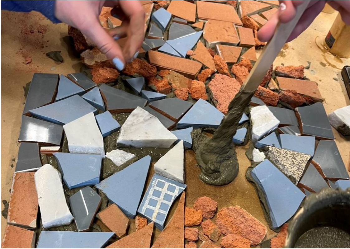
The materials are being glued to the substrate with high levels of precision. Photo: SINTEF
