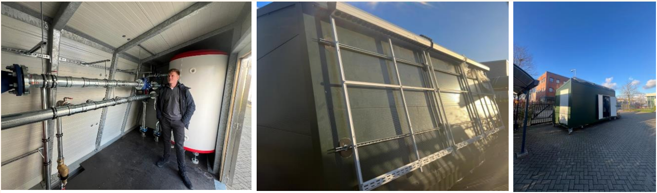
Figure 32 Pictures of the Bravo energy module as a key piece of the puzzle to create a sustainable apartmentbuilding
