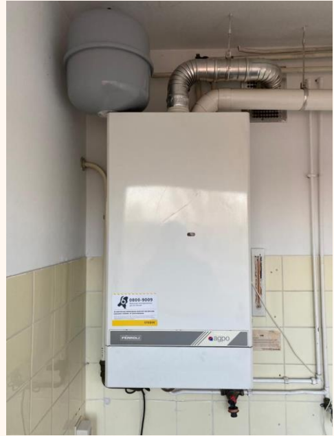
Figure 8. Current central heating boiler
